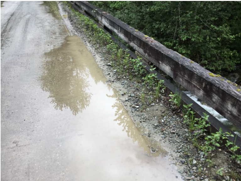
Sediment on deck
