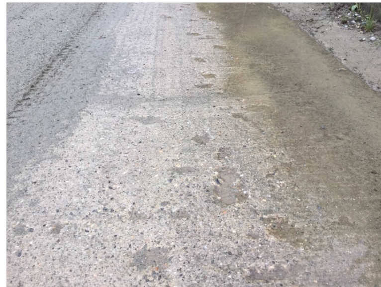
Minor damage noted on wheel path
