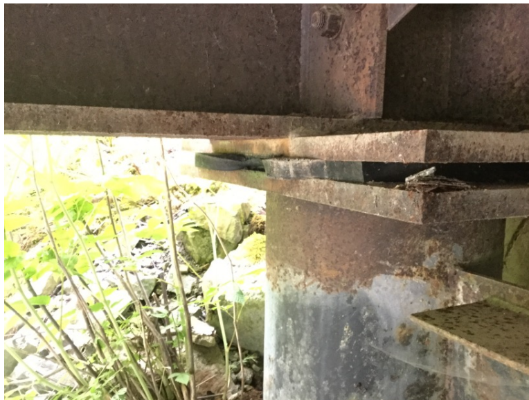
Typical bearing pad condition in all 4 cases
